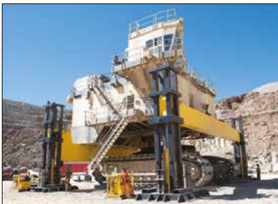
◀ A 1200-ton electric mining shovel being separated using custom 500-ton RR-Series cylinders and a pump per point synchronous lift system.
